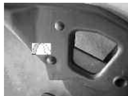
Lower rivet should be replaced with MS screw. (Aluminum rivet wears in steel lever and steel latch and allows lever to become loose and develop "wobble" which can lead to jammed flaps.)
